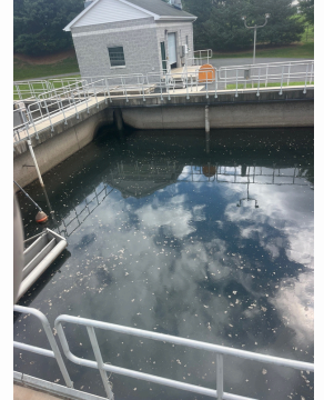
South Plant in anaerobic stage
