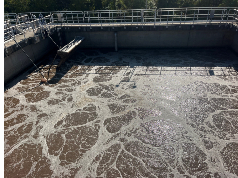
North Plant tank aerobic stage
